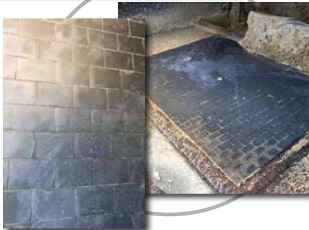
Transfer Hopper Wear Plates
